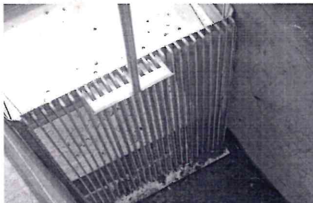
Figure 6 Screening at ETP Inlet
